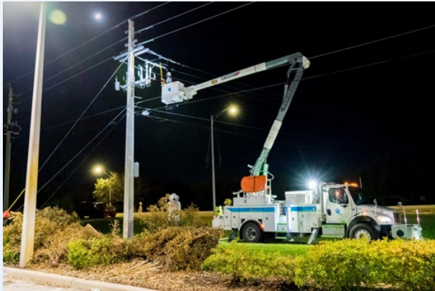
Our Terex Utility trucks operated day and night to restore the power grid.
